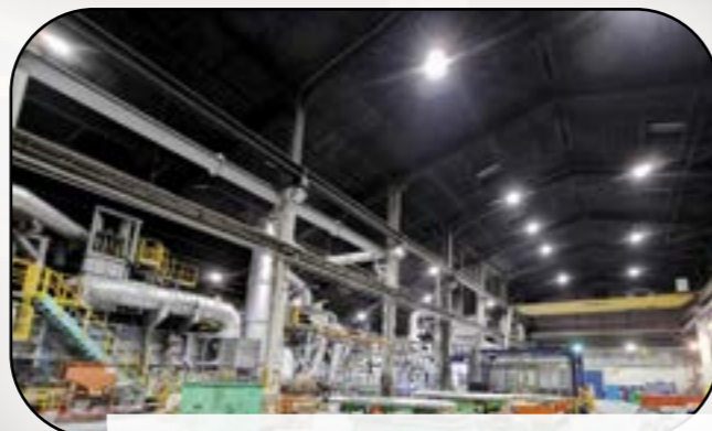
Relighting hall Hydro Aluminium
